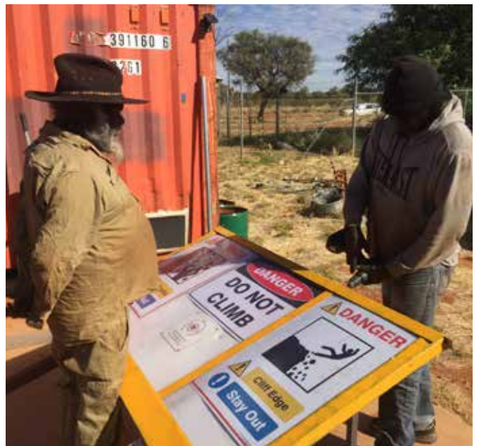
Mr Bennett blocking the Panel for Devon to insert the metallic sign frame.
